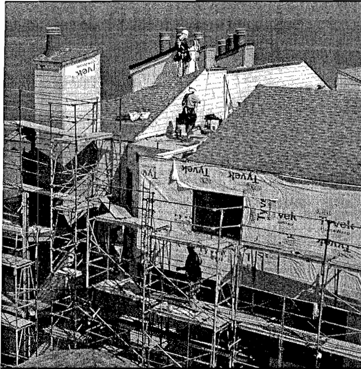
condominium complex in Solana Beach (above) is costing each owner about $100,000. "We are the prime example of deferred maintenance," Surfsong says. Acosta (below left) and Felix Lopez worked to repair a wall at San Carlos. Eduardo Contreras / Union-Tribune
